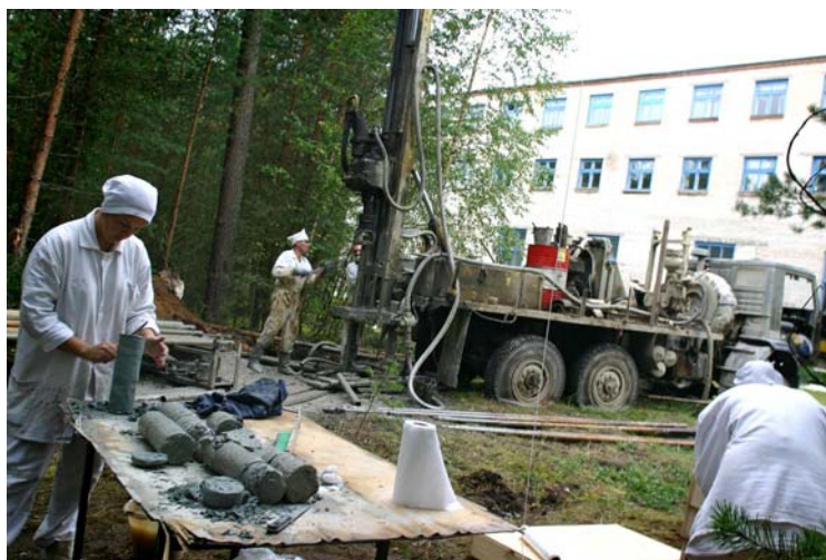
Figure 3: Core drilling and preparation of clay cores at RADON Sosnovybor (Saint Petersburg) (Figure 2 & 3 taken from V.G. Rumynin, et al. Research of Vendian and Cambrian clays as a medium for construction of a regional waste repository in N-W region of the Russian federation, The II International Forum, October 02-05 2007, Saint Petersburg)
